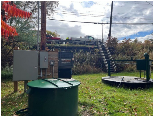
JHPS Control Panel, Wet Well, and Dry Pit
